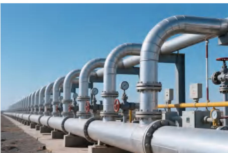
Oil Transmission Pipes
